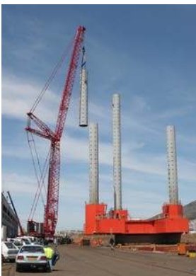
LEFT: Crane lifting the upper part of a leg of the jack-up rig.
